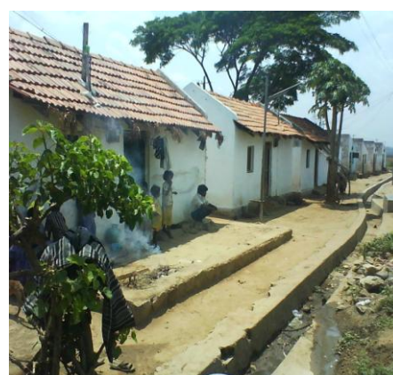
Drainage works carried out in N. Begur and Naganahalli panchayats under gram swaraj project under study.
